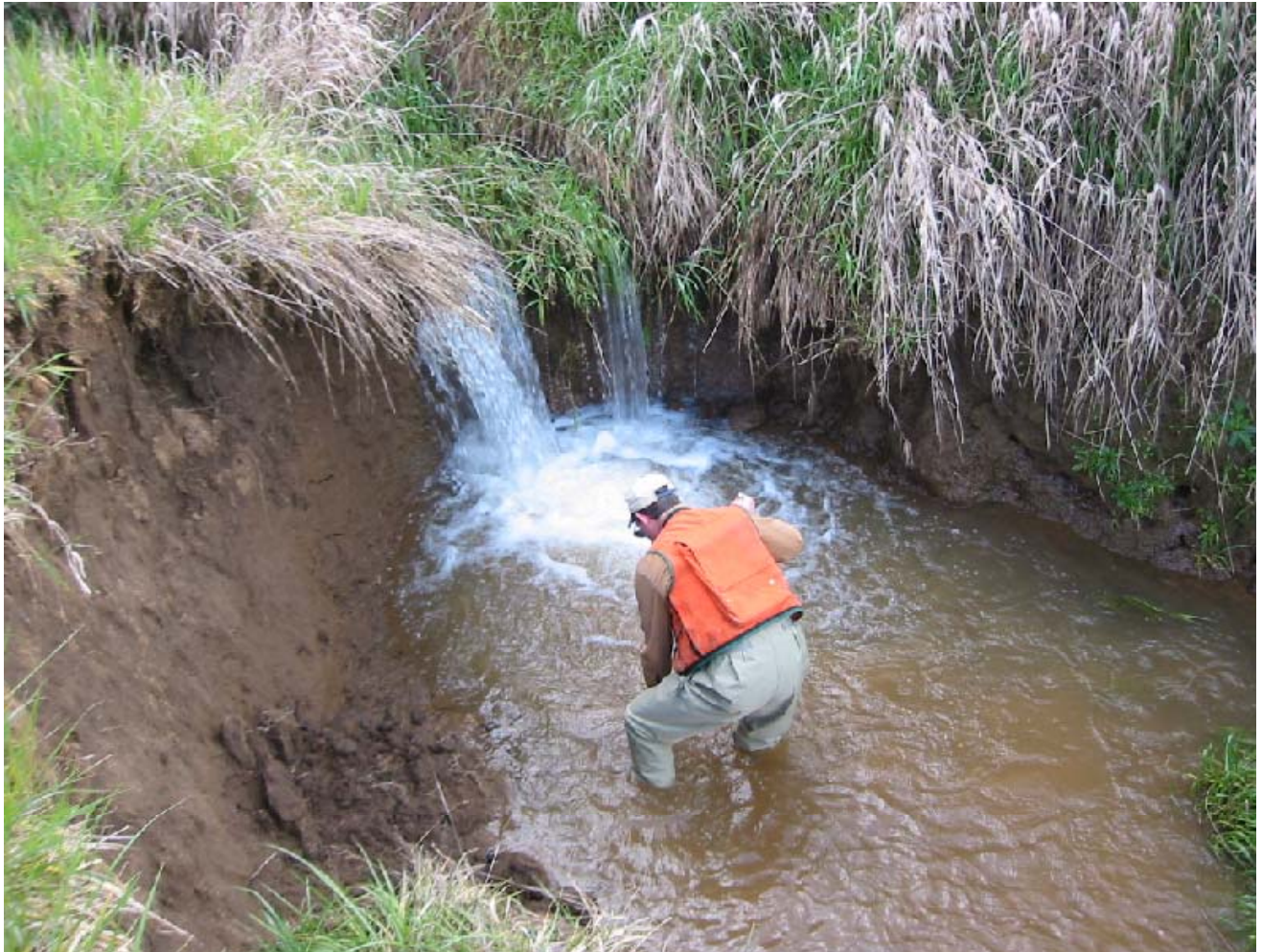
FIGURE 3. SLOUGHING BANKS AND HEADCUTTING APPROXIMATELY 100 FEET UPSTREAM OF THE CONFLUENCE WITH SCOGGINS CREEK.
