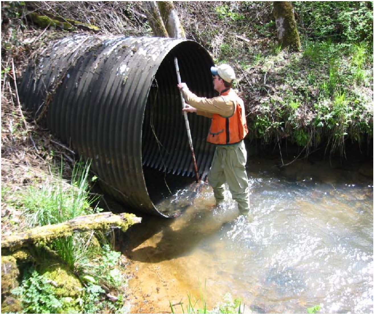
FIGURE 5. CULVERT AT THE SCOGGINS VALLEY ROAD CROSSING WITH A GRADIENT OF APPROXIMATELY 3 TO 4 PERCENT CREATING AN UPSTREAM PASSAGE BARRIER.
